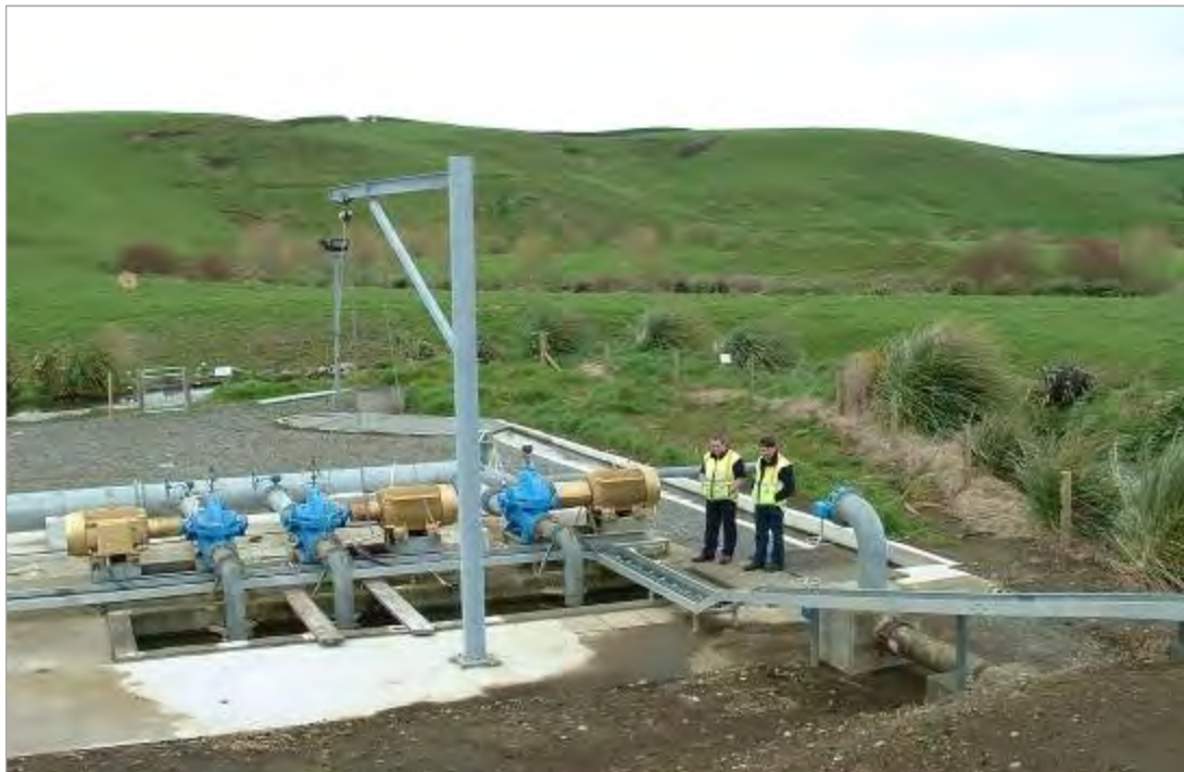
Photo 2 Tawhiti water intake
