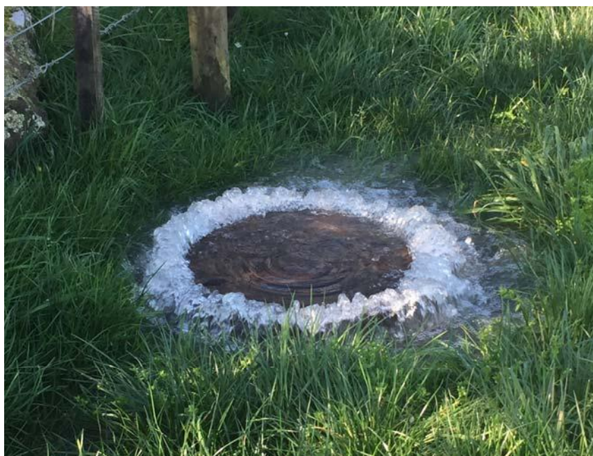
Photo 2 Motunui water take pipeline leak
