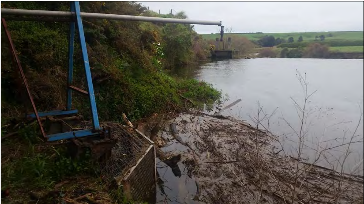
Photo 3 The intake and radar which records water level, showing a significant amount of debris accumulation, 21 September 2016
