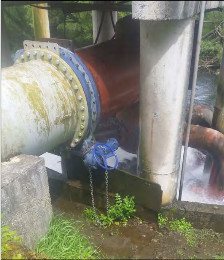
Photo 4 The control valve, unsecured during the inspection of 10 November 2016
