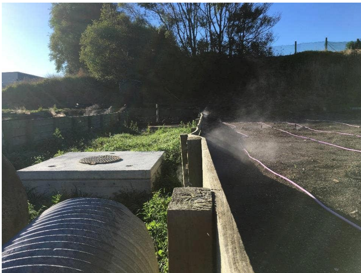
Figure 3: TBE concentrated sources biofilter inlet chambers and timber wall of the second bed.
