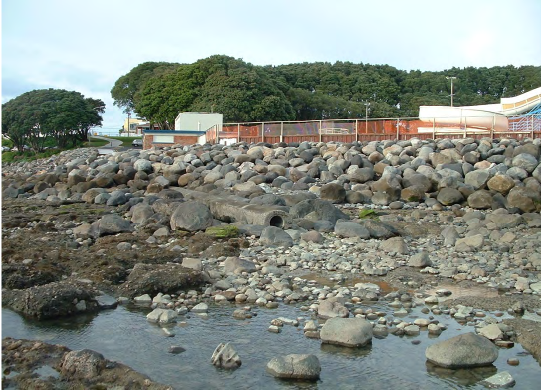
Photo 1 Aquatic Centre marine outfall
