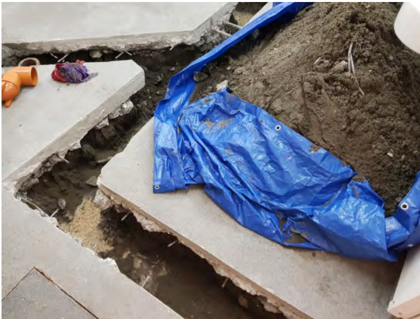
Photo 3 Extensive works being undertaken by NPDC to divert greywater from the women's showers to the sewerage system
