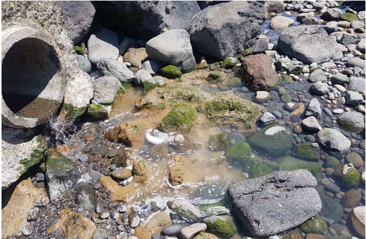
Photo 2 Foam discharging from outfall
