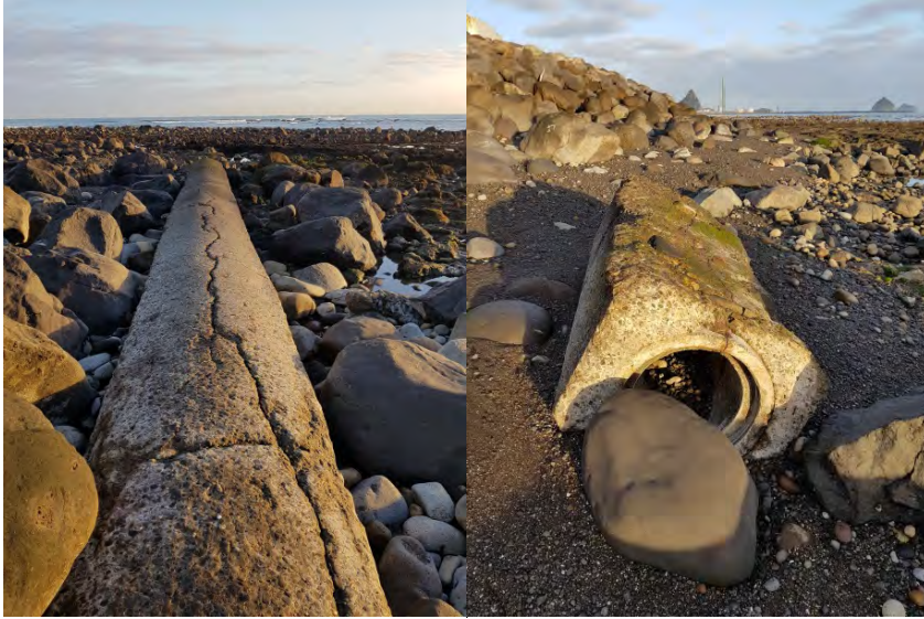
Photo 2 Cracks visible on the surface of the marine outfall structure (left), and the 2.4 m length of pipe dislodged from the end of the pipe at the Aquatic Centre (right)
