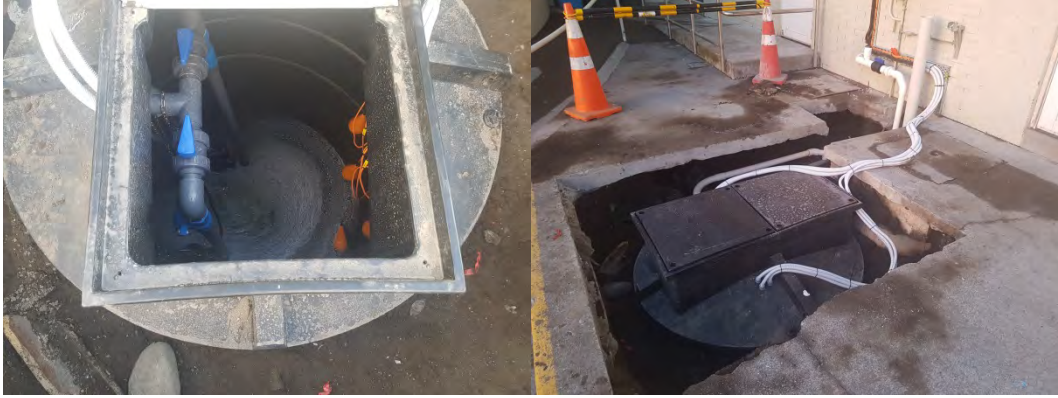
Photo 4 Commissioned works undertaken at the Aquatic Centre to divert greywater from the women's showers to the sewerage system (photo courtesy of NPDC, 27 June 2017)
