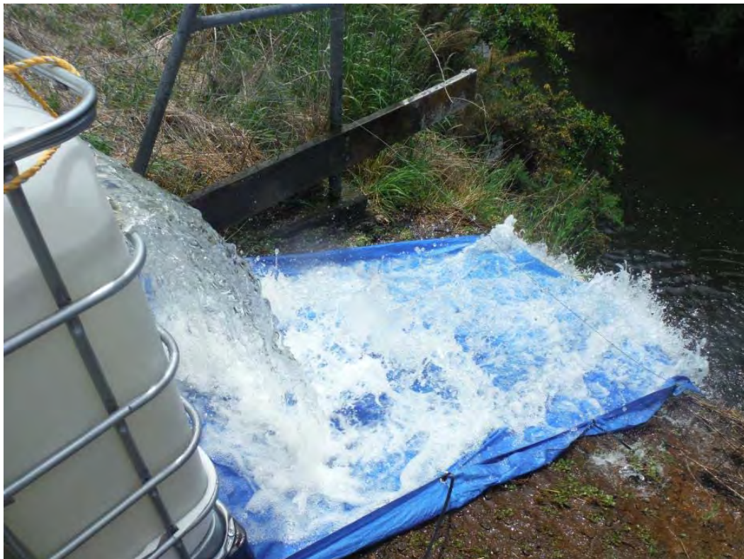
Figure 4. Water emptying from top of container onto sheeting used to prevent scouring
