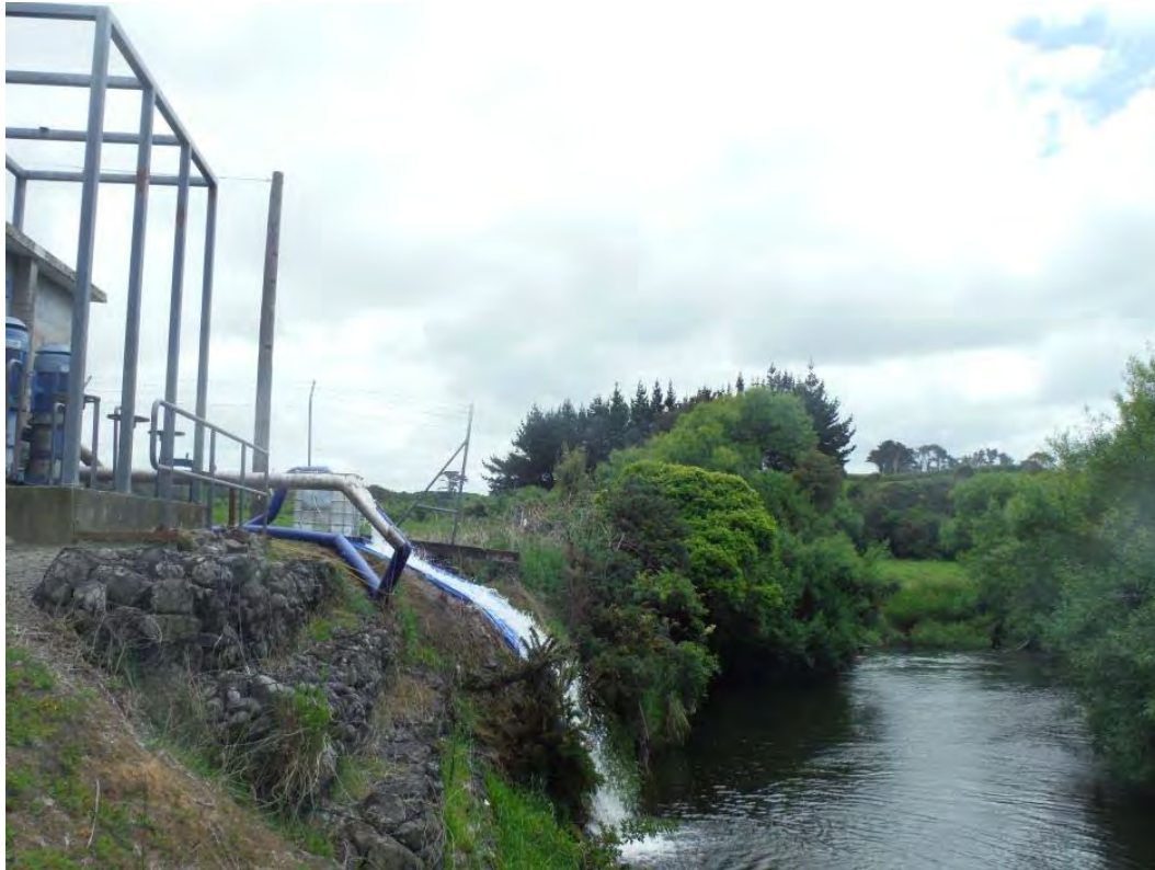
Figure 5. Overview of sampling operation with the pumps and other infrastructure to the left hand side of the picture
