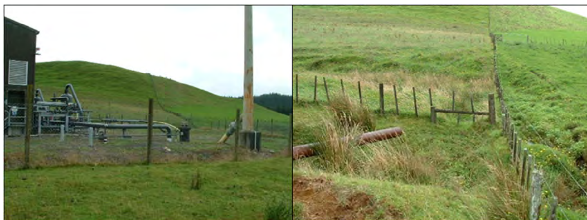
Photo 3 Ahuroa B site looking towards the skimmer pit (left) and the final discharge point
