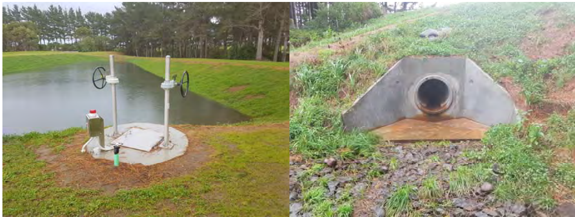
Photo 2 Northern stormwater pond, stop valves and outfall to the Kaipokonui Stream
