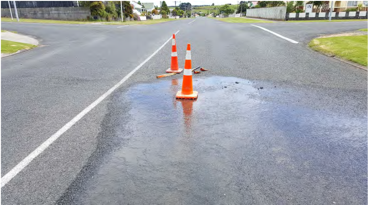
Photo 6 Wastewater discharge to stormwater (Incident IN/35450)
