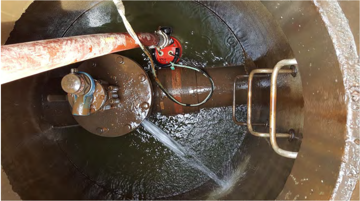
Photo 5 View of the wastewater leak at the PSV (Incident IN/35450)
