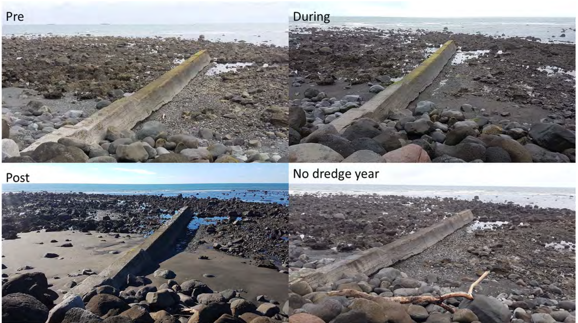
Figure 12 Looking north at the groyne on Arakaitai Reef from the walkway; pre (6 Jan 2017), during (17 Feb 2017), and post (10 Apr 2017) dredging campaign and the following year (28 Mar 2018)
