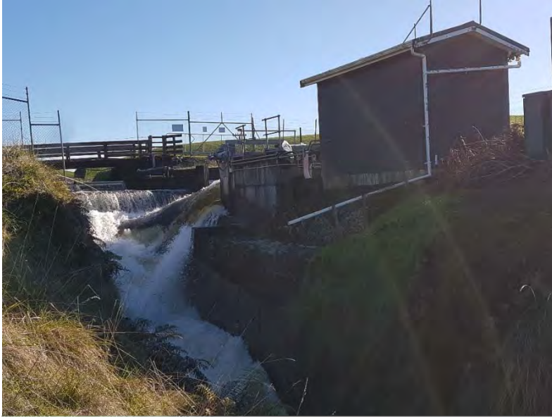
Photo 4 In race generator, 27 June 2018
