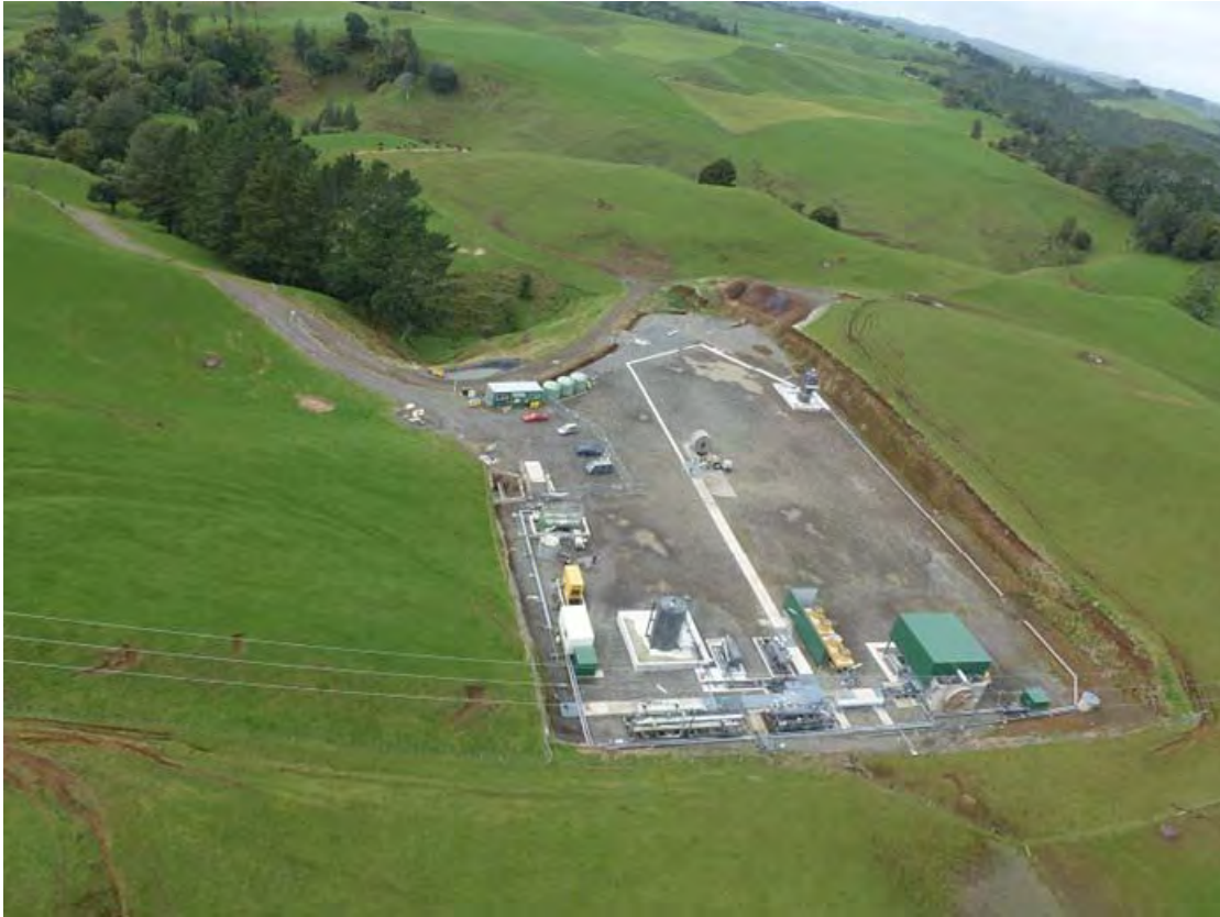
Photo 2 Kowhai-A Production Station
