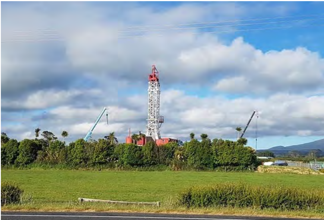
Photo 2 Radnor Production Station
