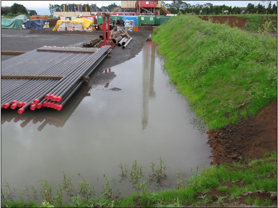
Photo 1 Substantial ponding seen overflowing the ring-drain at the Kowhai-C wellsite on 5 December 2013
