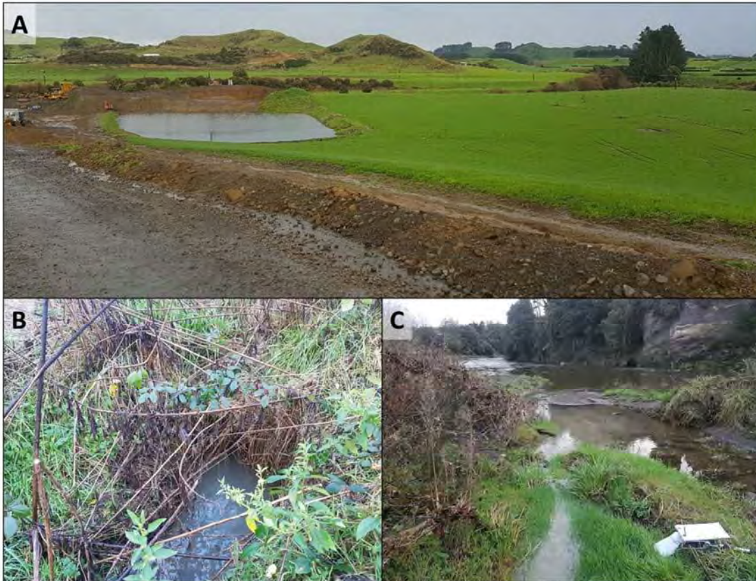
Photo 2 A: Pond conversion and reinstated paddocks. B: Settlement pond discharge point. C: Discharge mixing with Patea River.
