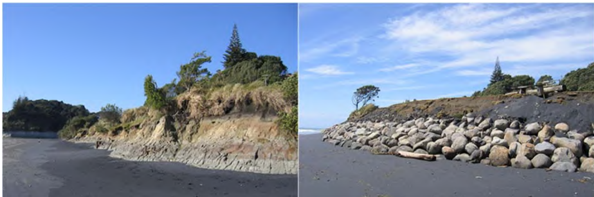
Photo 2 a) Erosion on Wai-iti foreshore prior to construction of the rock wall and b) rock wall facing north from stream (Nov 2005)
