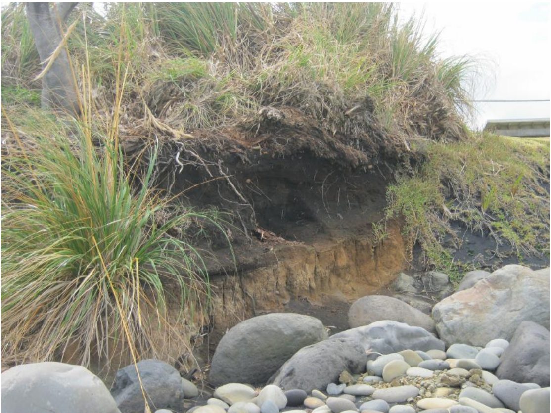
Photograph 6 Erosion along the top of the rock wall
