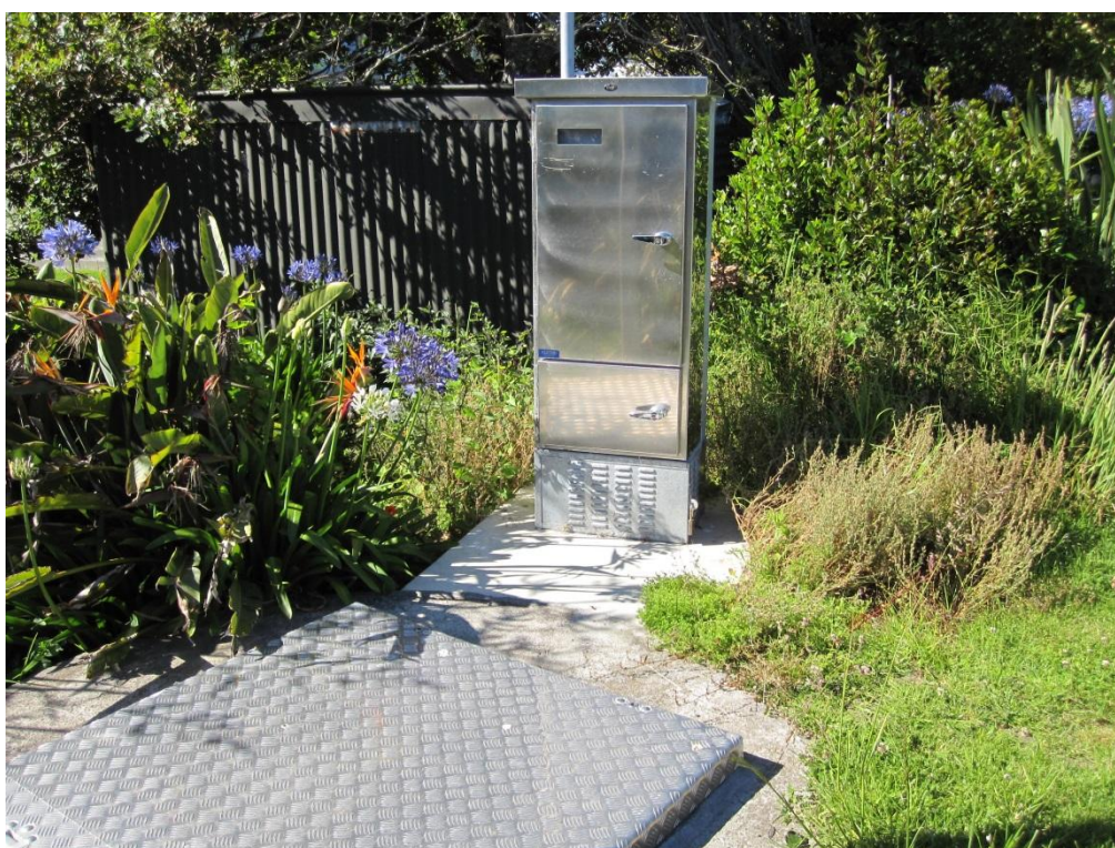
Photo 6 Improvements to pump station including new lid, switchbox and alarm system (20 December 2013)
