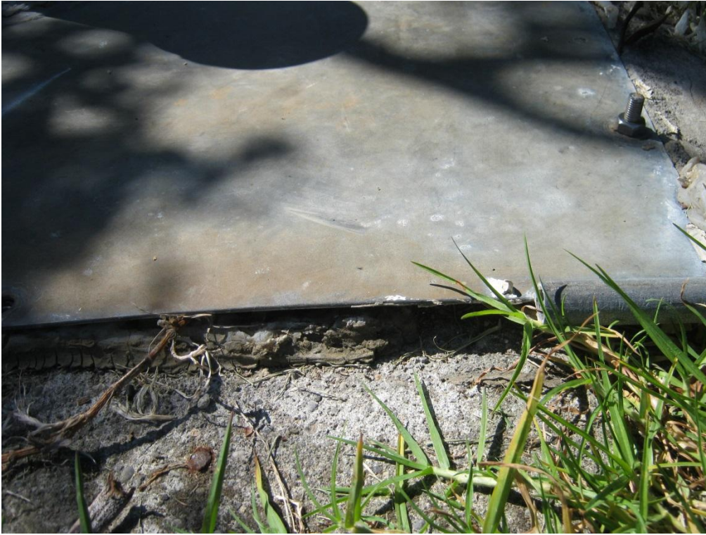
Photo 4 Gaps around the pump station (lid 29 January 2014)
