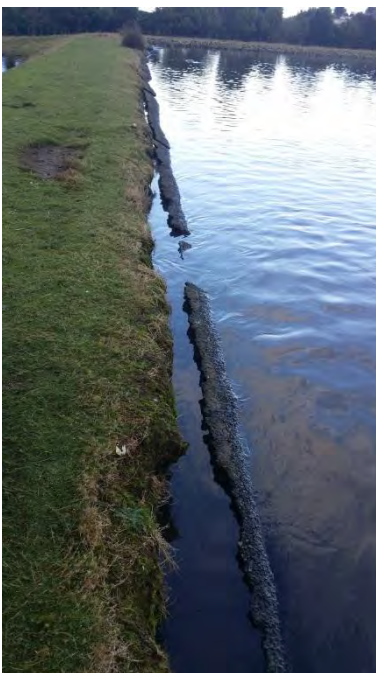
Photo 3 Waveband erosion June 2015
