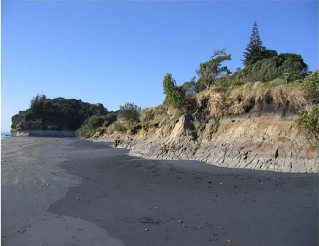
Photo 3 Erosion on Wai-iti foreshore prior to construction of the rock rip rap seawall
