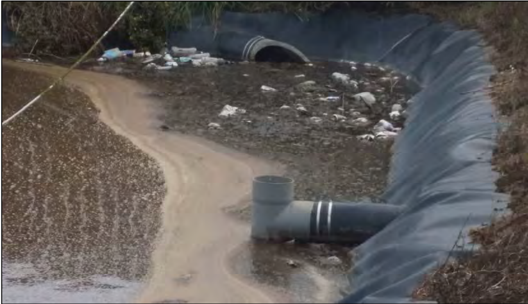
Photo 1 Floatables on the Waverley stock truck wastes Pond 1, February 2016
