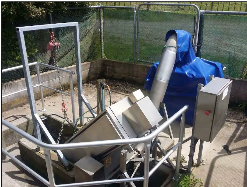
Photo 2 Step screen facility at the inlet to the Stratford WWTP.
