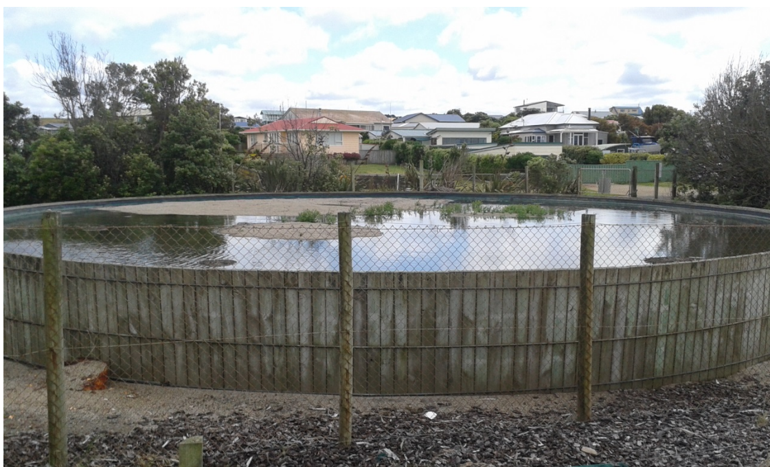
Photo 1 Wastewater ponding and weed growth on the surface of the eastern filter bed, 21 December 2015
