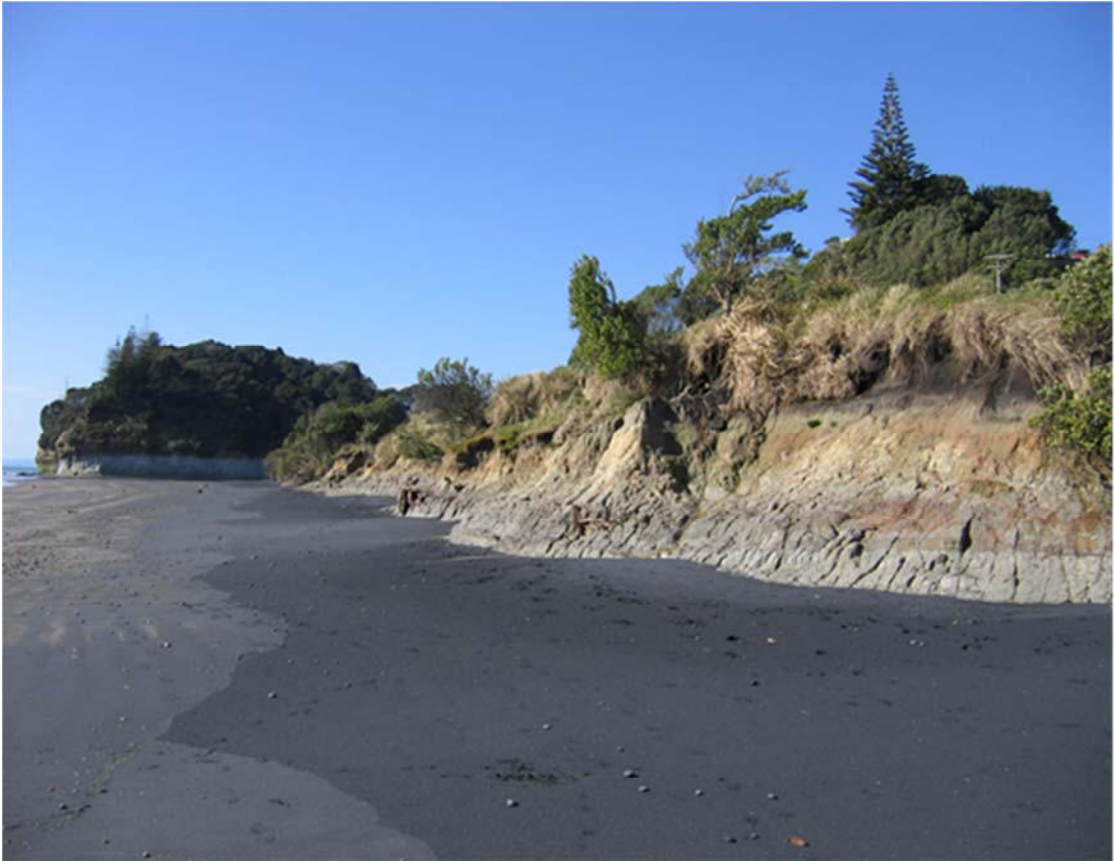
Photo 3 Erosion on Wai-iti foreshore prior to construction of the rock wall
