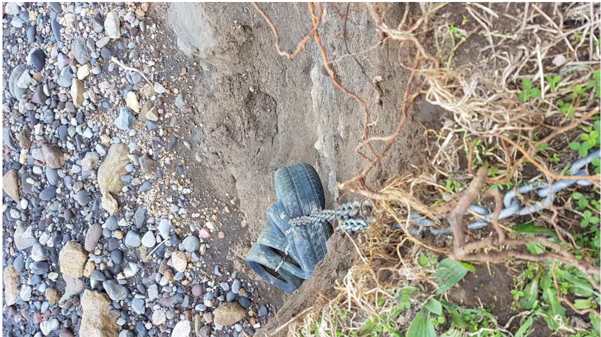
Photograph 5 Tyre ladder following slip June 2017
