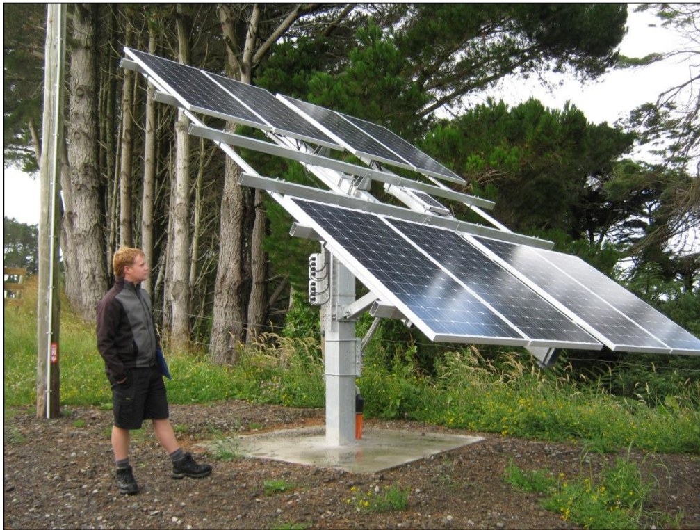
Photograph 7 Solar panel array powering Mangawhero-iti intake data logging and telemetry
