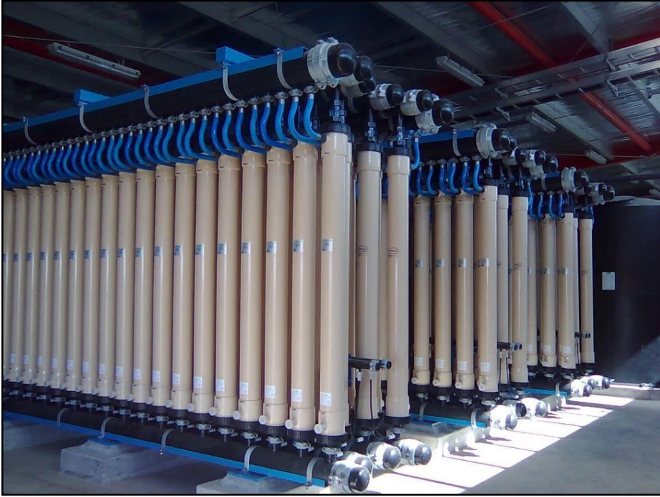
Photograph 1 Membrane racks at the new Kapuni WTP
