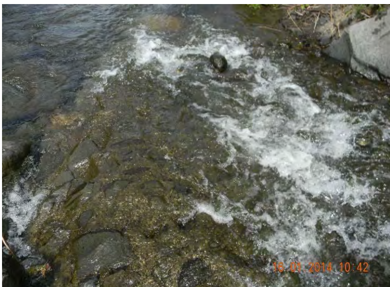
Photo 3 The lower section of the fishpass showing where the large rocks have been sheared off
