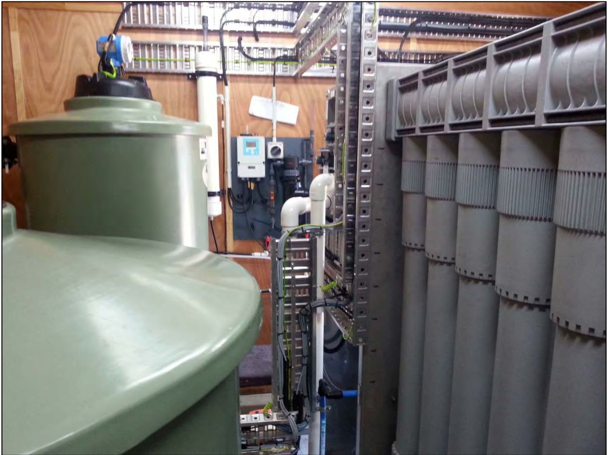
Photo 1 New membrane filters at Rahotu WTP
