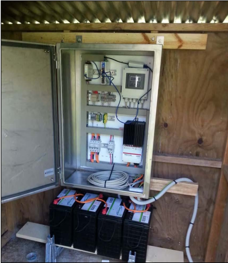
Photograph 1 Upgrade data shed at Mangawhero take
