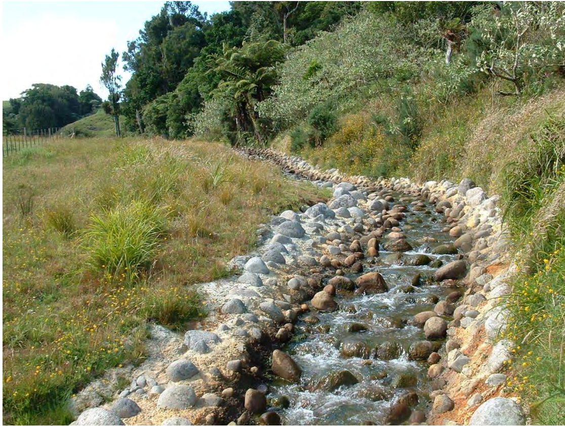
Figure 1 Kakapo Stream looking upstream, approximately half way up fish pass over the former Urenui water supply dam
