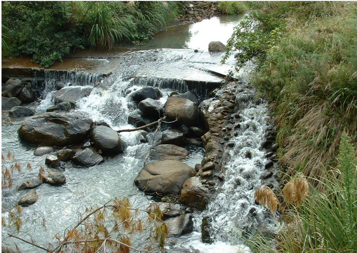
Photo 1 STDC weir, new fish pass (right of photo) and old fish pass (left of photo) in the Mangawhero Stream
