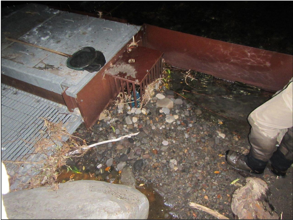
Photo 3 The inlet to the fish pass blocked by gravels, 20 April 2016.
