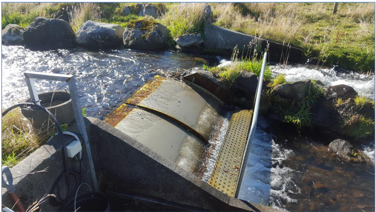
Photo 1 CCCWSL's weir and intake screen
