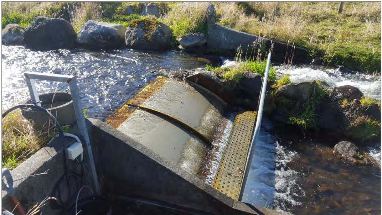
Photo 1 CCCWSL's weir and intake screen
