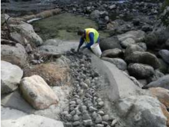
Photo 2 TRC biologist placing rocks in the steepest section of the new fish pass
