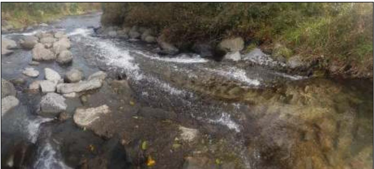
Photo 3 The fishpass showing where the large rocks have been sheared off (24 April 2018)
