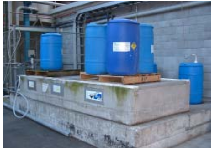
Photo 1: Large quantities of chemicals should be stored in bunded areas
