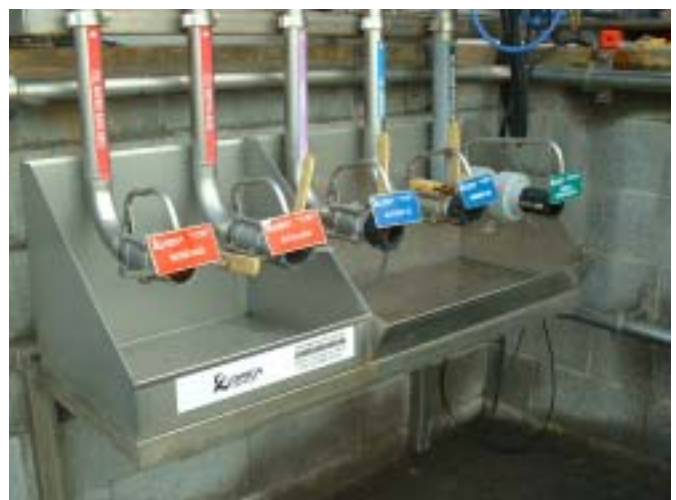
Photo 2: Secondary bunding within a bunded area
