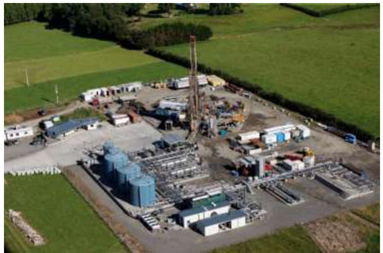
Photo 2 Drilling rig (background) and production facilities (foreground) at the Cheal A wellsite/production station, Taranaki
