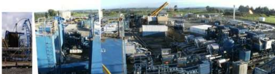
Photo 5 New Zealand wellsite - Mangahewa wellsite photographic mosaic showing from left to right coil tubing, storage tanks and pump trucks around the wellhead, gas processing equipment, and flare pit (Source: Boeren, 2011)
