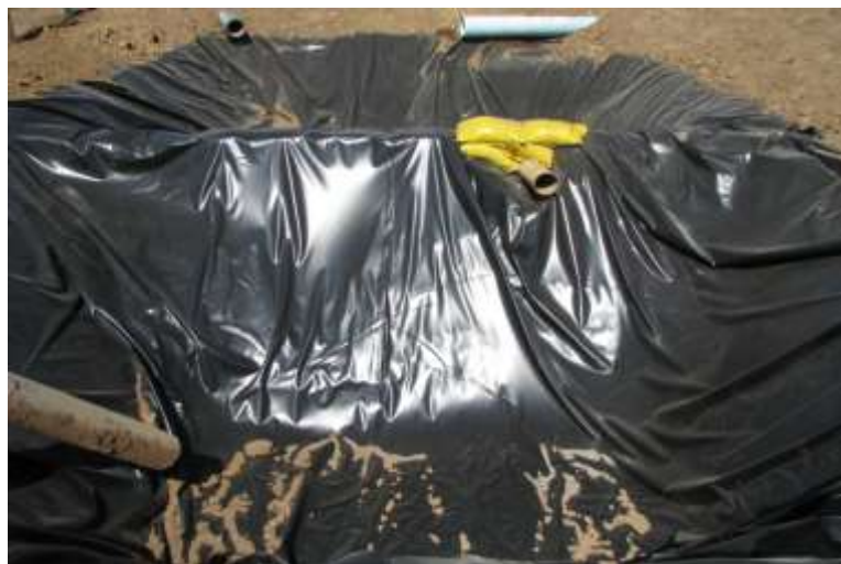
Photo 14 Wellsite skimmer pit with site stormwater entering the lined pit and a "goose neck" pipe exiting the pit
