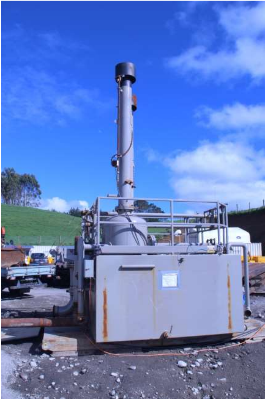
Photo 13 Cheal B wellsite thermal oxidiser (flare box)
