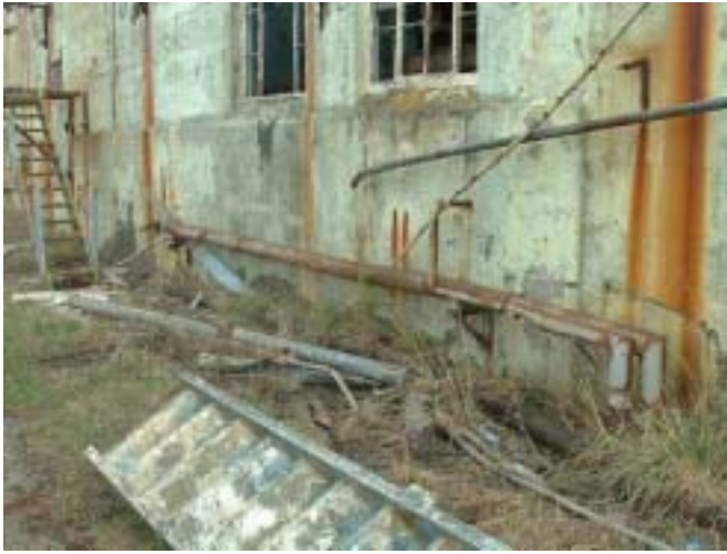
Photograph 6 Fuel oil pipework into the Boiler House
