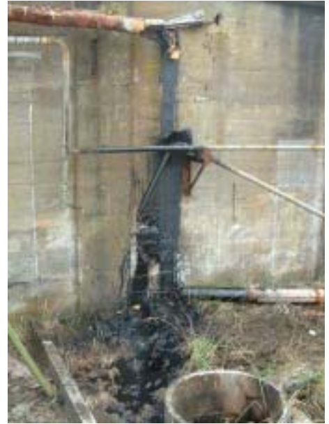
Photograph 7 Leaking fuel oil
