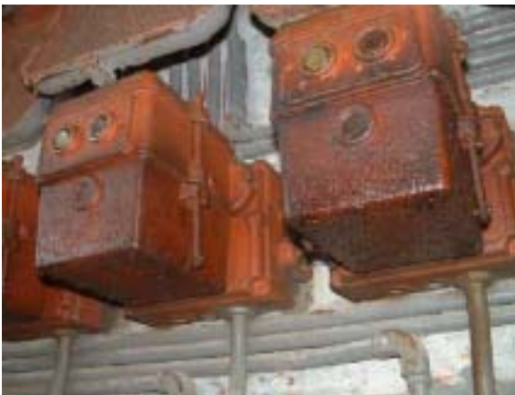
Photograph 13 Electrical equipment containing PCBs remaining on site
