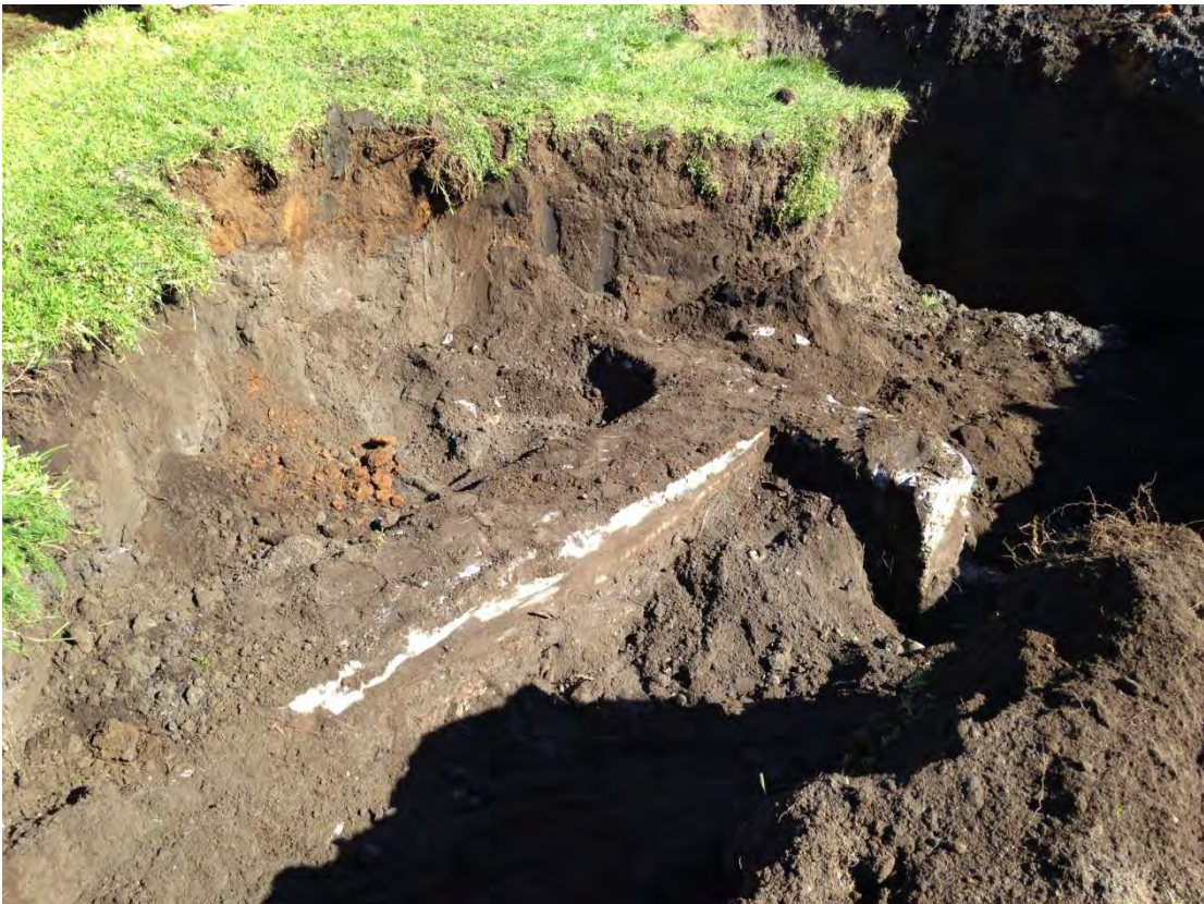
Photograph 18: Large concrete footing, likely associated with a former pumpjack, identified in test pit TP14.
