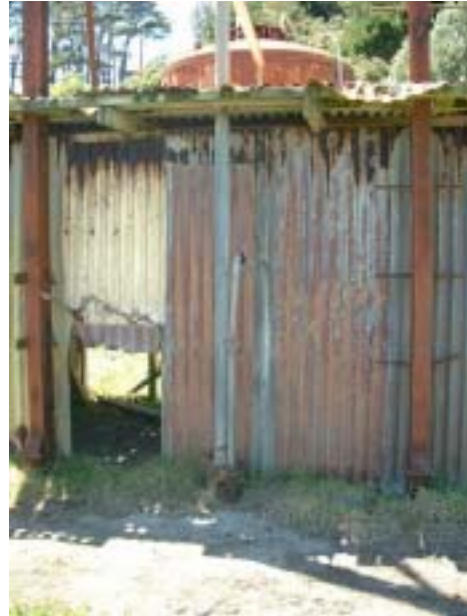
No. 8 well pumpshed
