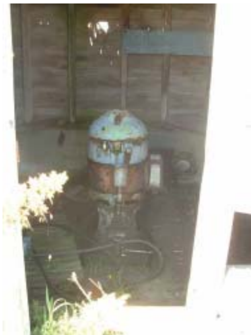
No. 1 well pump
