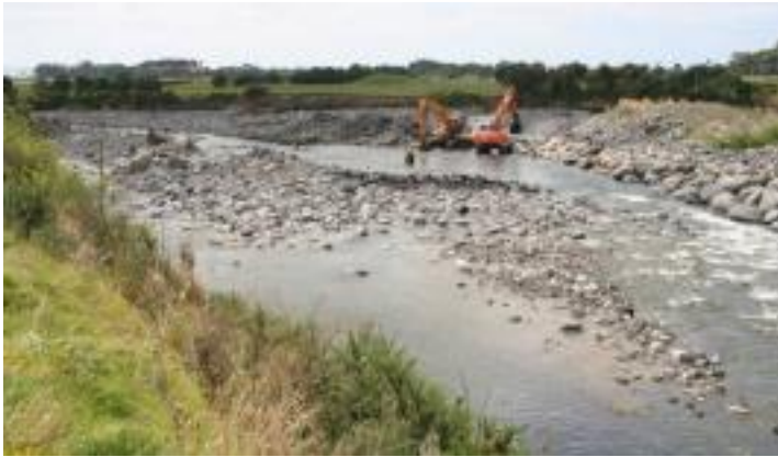
Photo 14 Stony River – Establishing a diversion cut to re-align a channel through an aggraded area
