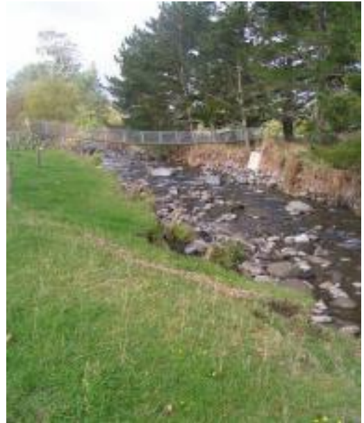
Photo 2 Kaihihi Stream – Stony Walkway - bridge closed by bank erosion
