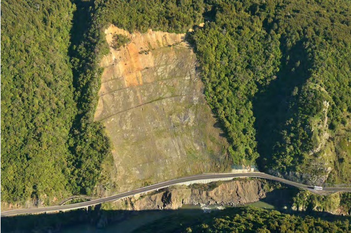
Figure 35 Head scarp failure of pre-existing landslide in Manawatu Gorge. The landslide had been benched and drainage installed following major failures in 2004 and 2011. (GNS Photo: D02_1859)
