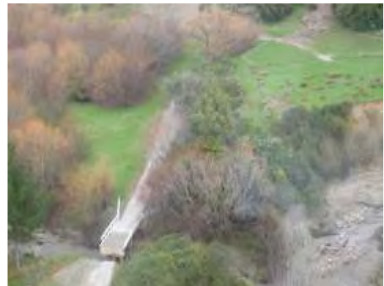
Photo 17: Makakaho Rd, damaged bridge
