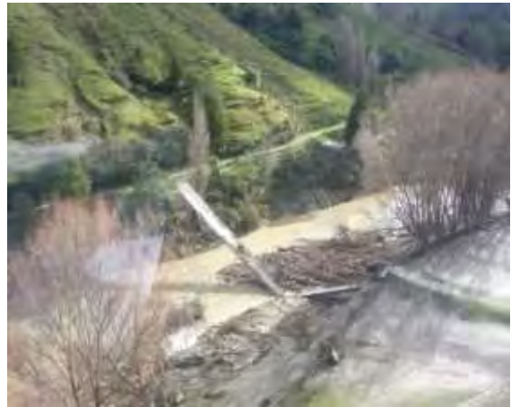
Photo 10: Damaged bridge on Puao property, Waitotara Valley Rd
