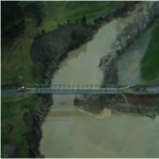
Photo 25: Damage to Limestone Bridge, Waiinu Beach Road , Waitotara
