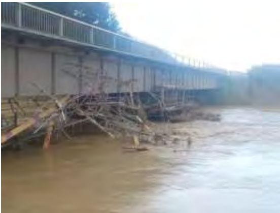
Photo 26: Damage to scaffolding on Waitotara SH3 Bridge Waitotara
