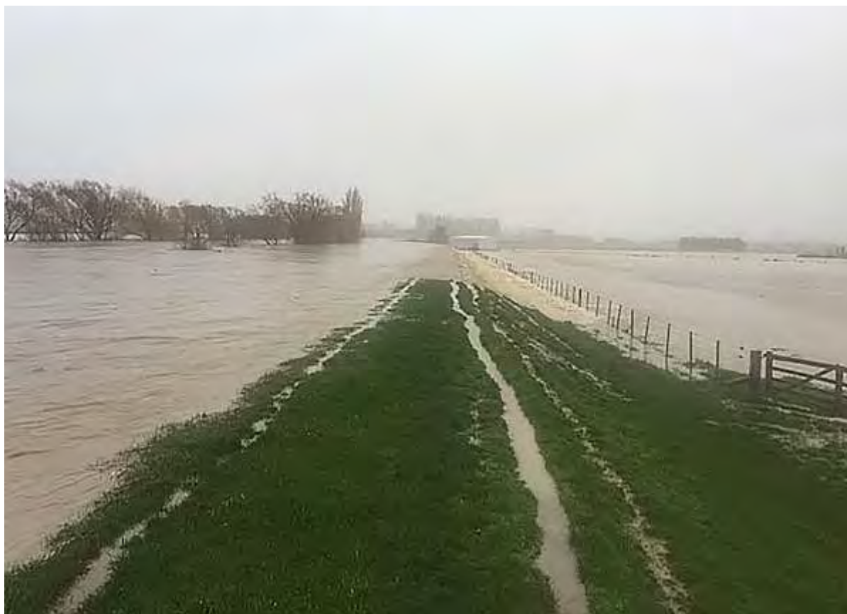
Photo: Selwyn River stop-bank overtopping in July 2017.
