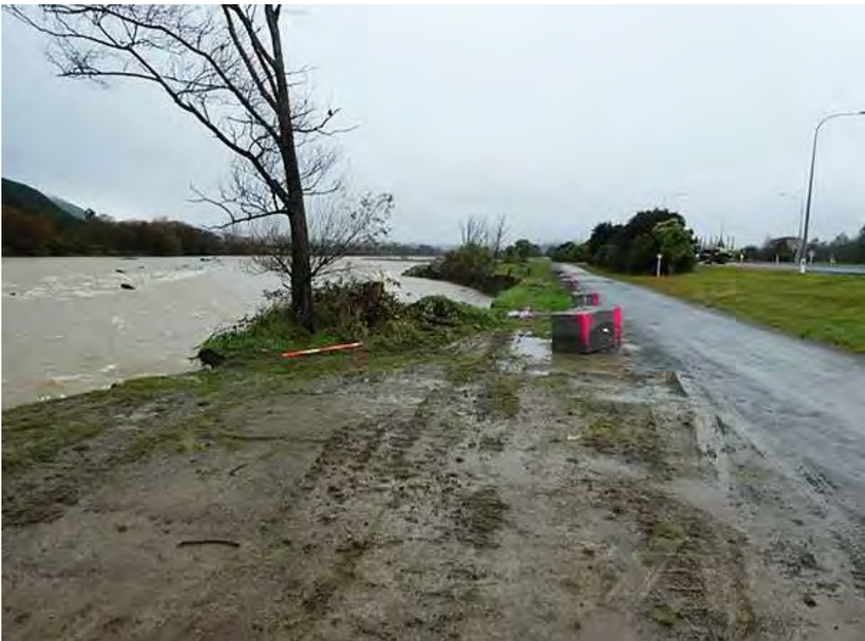
Hutt River erosion adjacent to State Highway two during a small annual flood event in June 2018
