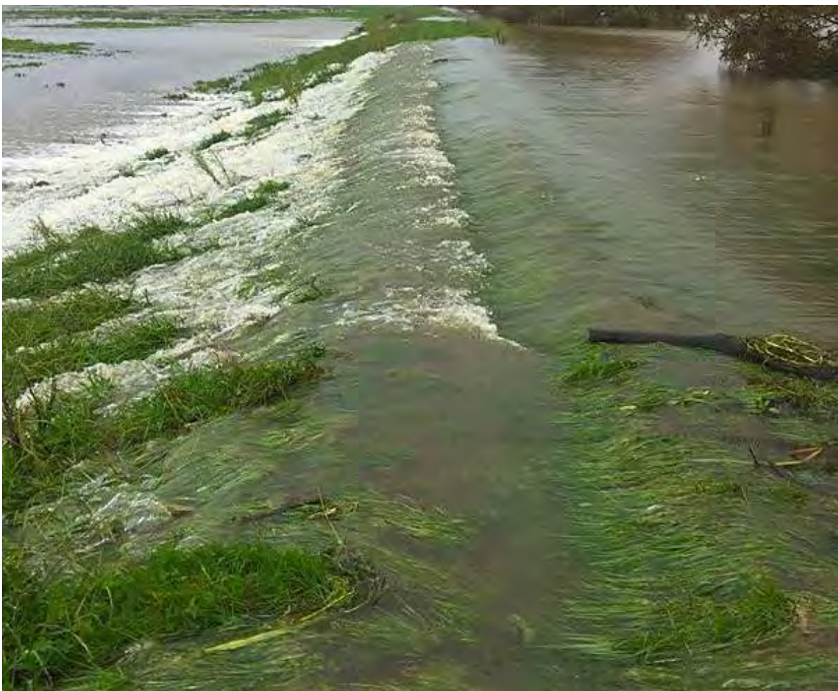
Overtopping of the stop-banks and inundation of Hauraki Plains by the Piako River flood in April 2017 (NB This 100-year flood event far exceeded the 50-year flood-event design capacity of the existing scheme).
