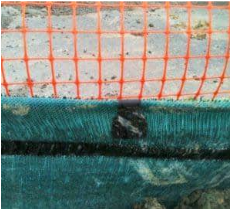
Silt fence correctly secured to the top wire using silt fence clips (Source: SouthernSkies).
