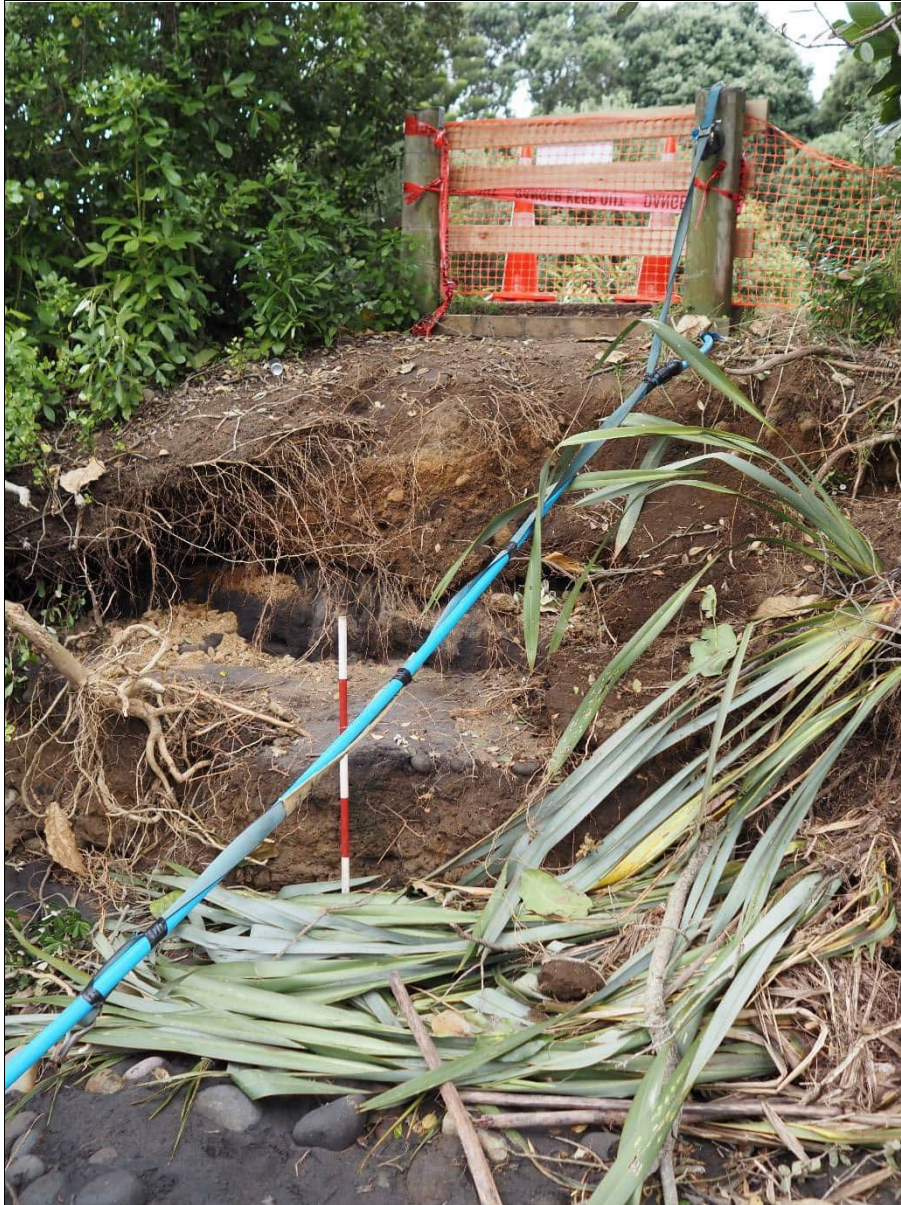
Figure 7: Site P19/422, Oven stones exposed below washed-out bridge foundation in February 2022 (Image: Ivan Bruce, February 2022).
