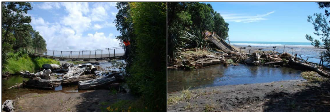
Figure 1-4: Before the existing bridge failure (left) and post-failure (right) (image from WSP, 2023).
