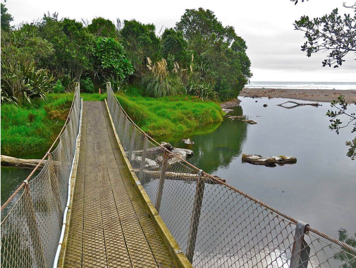
Figure 24 Photograph looking west from Ahu Ahu road across the previous swing bridge (now destroyed) towards site of proposed shared pathway.
