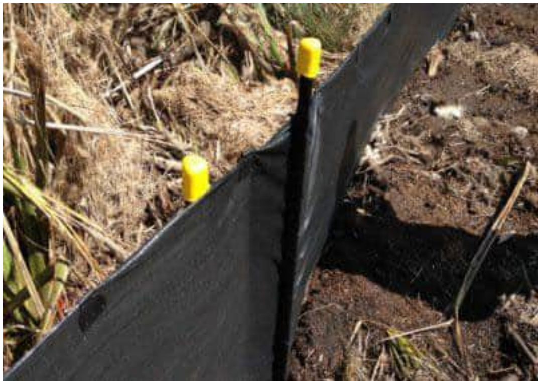
Doubling the fabric over at the end around the waratah (Source: SouthernSkies).
