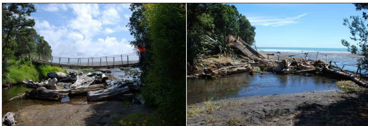
Figure 2.9: Images of before the existing bridge failure (left) and post-failure (right). (Source: WSP, 2023).
