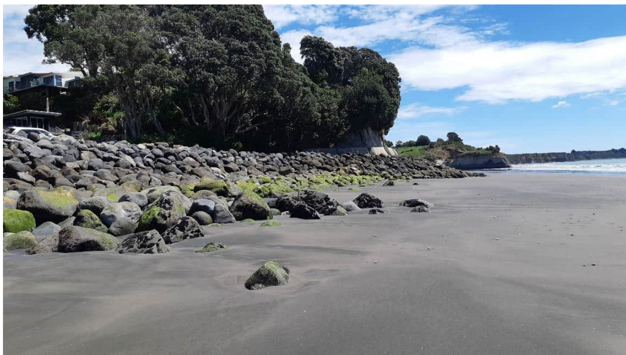
Figure 13 Photograph showing rock revetment along New Plymouth coastal walkway with backdrop of vegetation.
