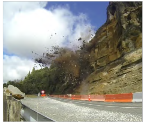
Blasting as part of rock stabilisation works at Mangaotaki Bluffs in May 2014
