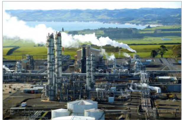
Motunui methanol plant on SH3 north of New Plymouth
