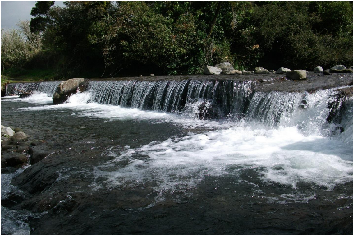
Long disused farm access ford in Kapuni Stream downstream of Opunake Road that needs removing.
