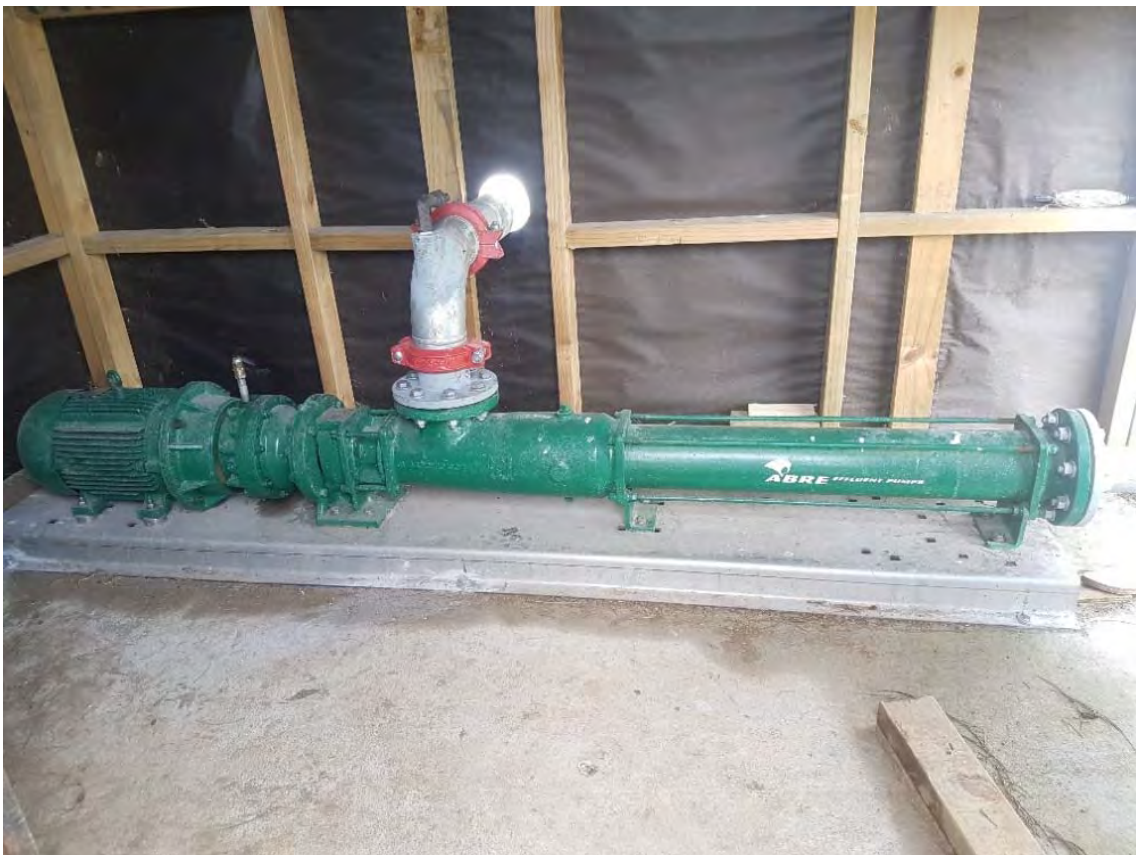
Figure 12 Inside the pump shed showing the multi stage variable speed pump
