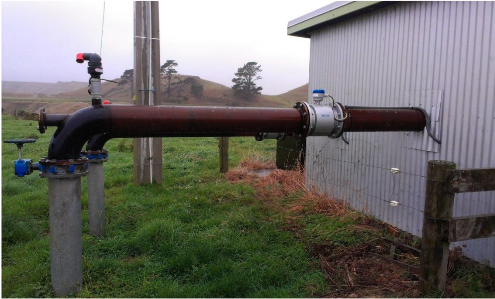
Photo 5 Good installation of a flowmeter
