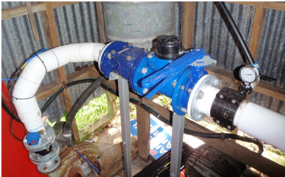
Photo 6 Poor installation of a flowmeter
