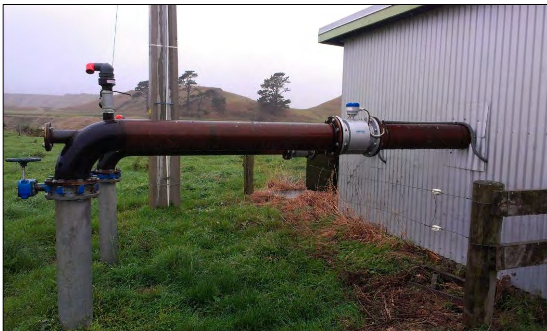
Photo 5 Good installation of a flowmeter
