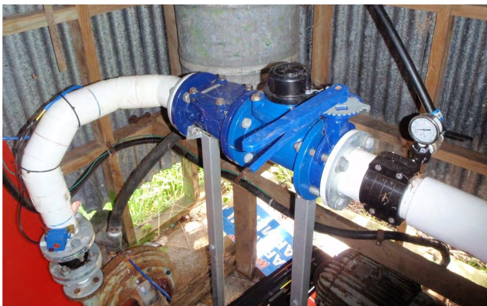
Photo 6 Poor installation of a flowmeter
