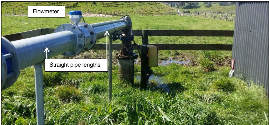
Photo 4 Good installation of a flowmeter
