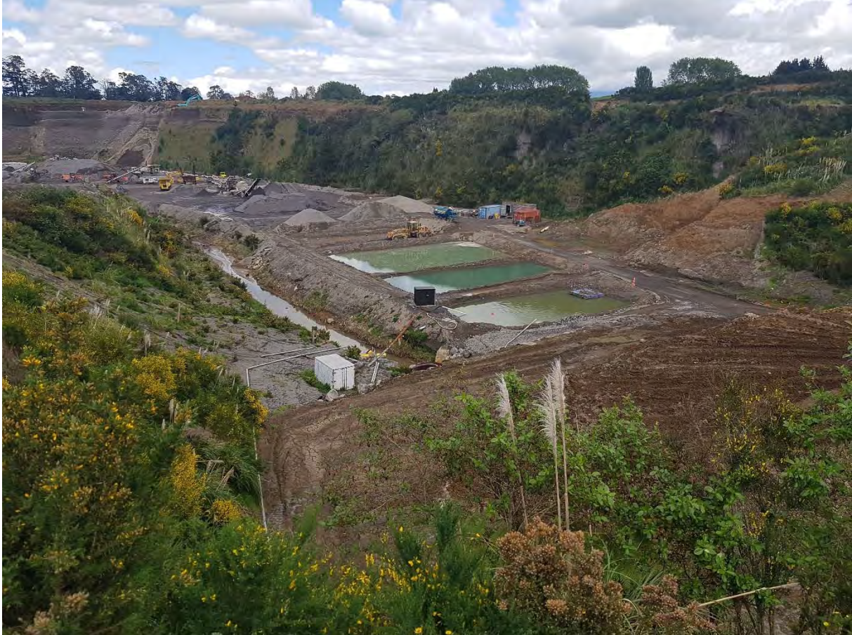
Photo 1 Everett Road Quarry view from upper pond area, looking at new washwater treatment ponds and active excavation area.
