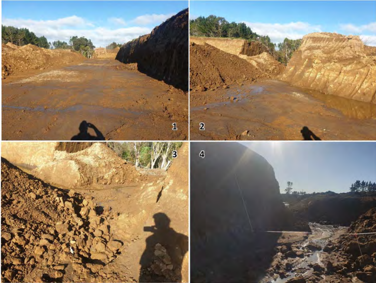
Photo 7 The majority the site (1) is directed straight to the discharge (2 & 3) point without treatment (4).
