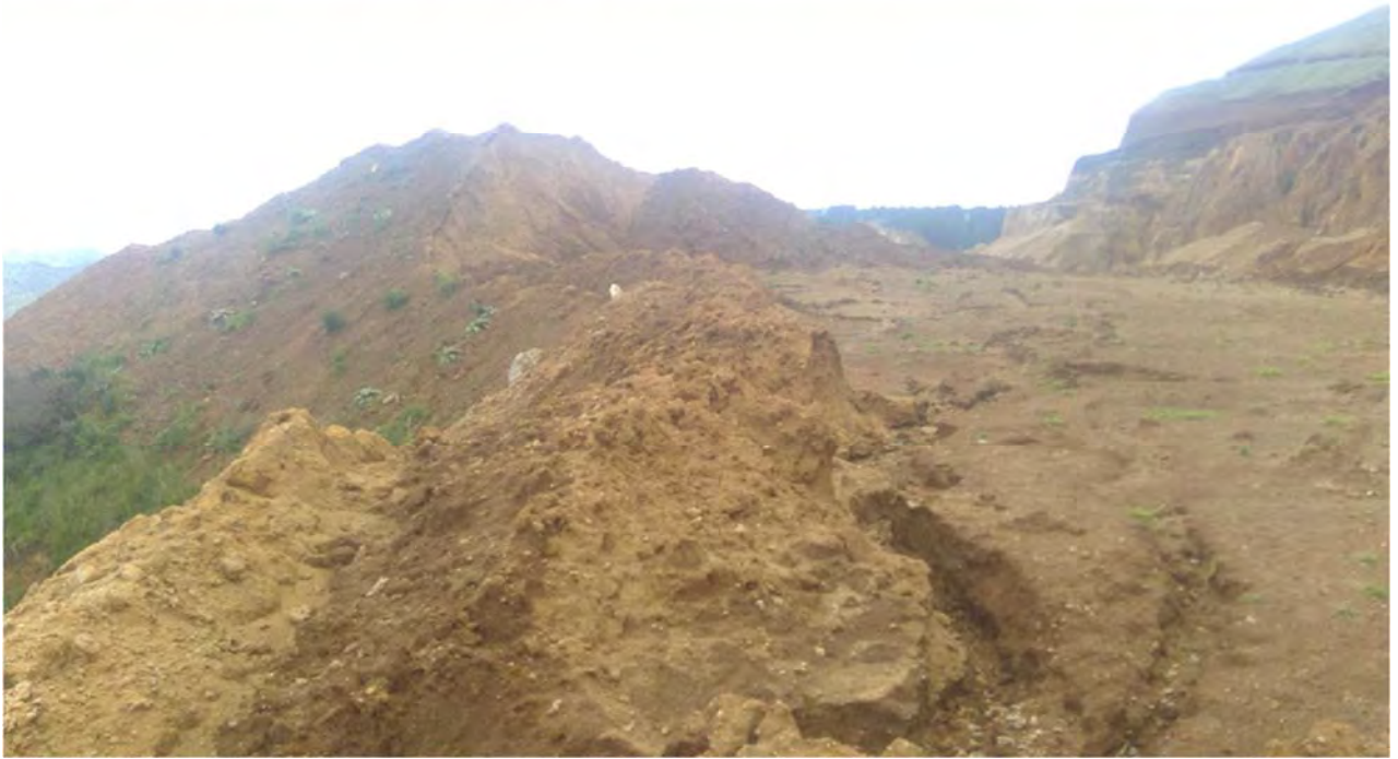
Photo 10 Contouring in the top photo directs water directly off the back of the site without treatment shown in the bottom photo. December 2019
