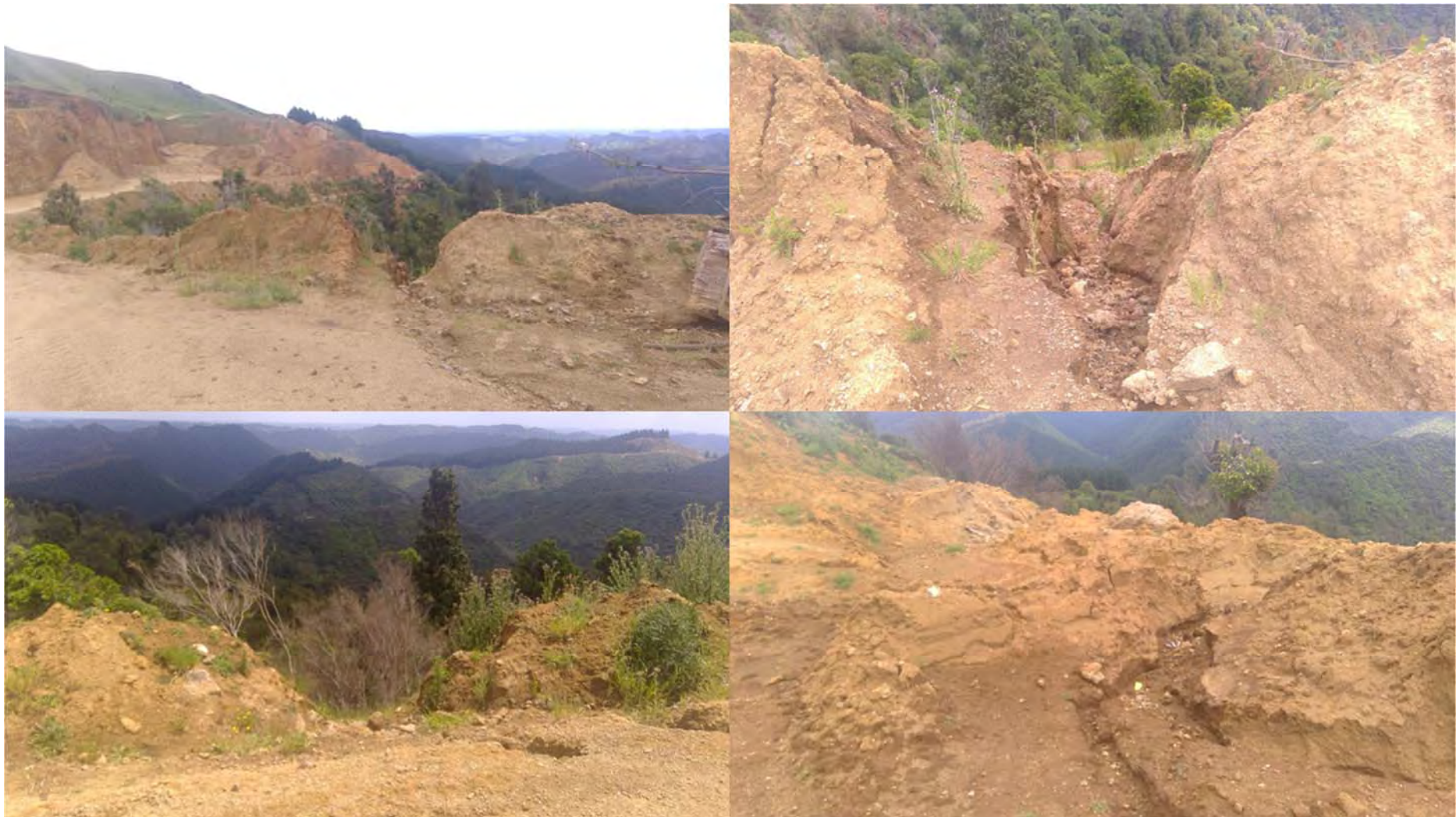
Photo 9 Examples of bunding failures and erosion throughout the site December 2019 allowing runoff to escape before treatment
